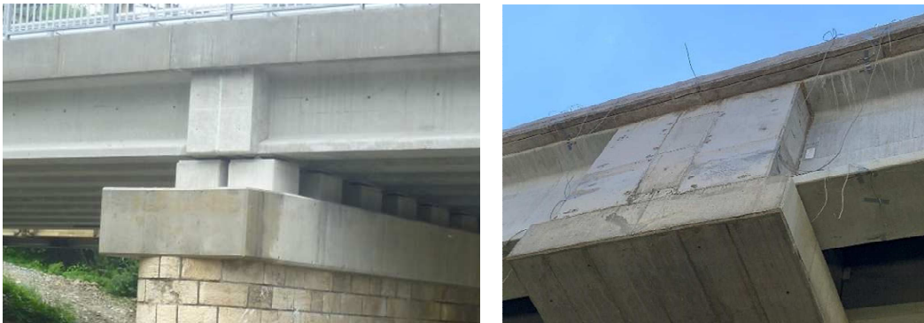
Fig. 1: Detail over the pier: simply supported spans with continuous slab (left), full continuity (right).
