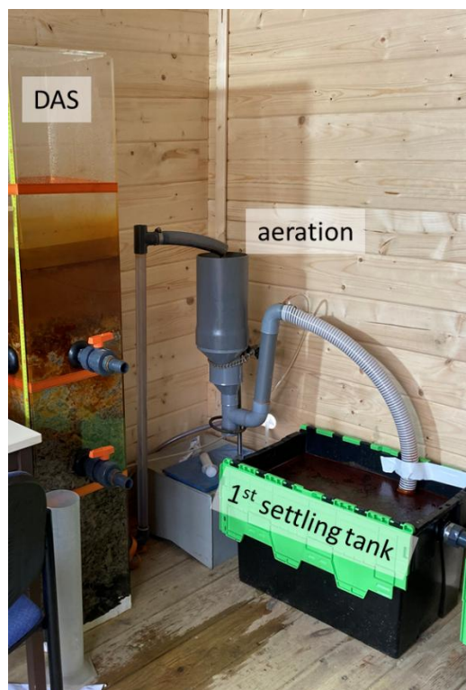
Figure 1. AMD pilot plant on site
