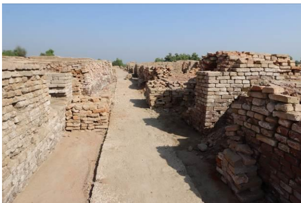
Path blocking run-off, HR area
