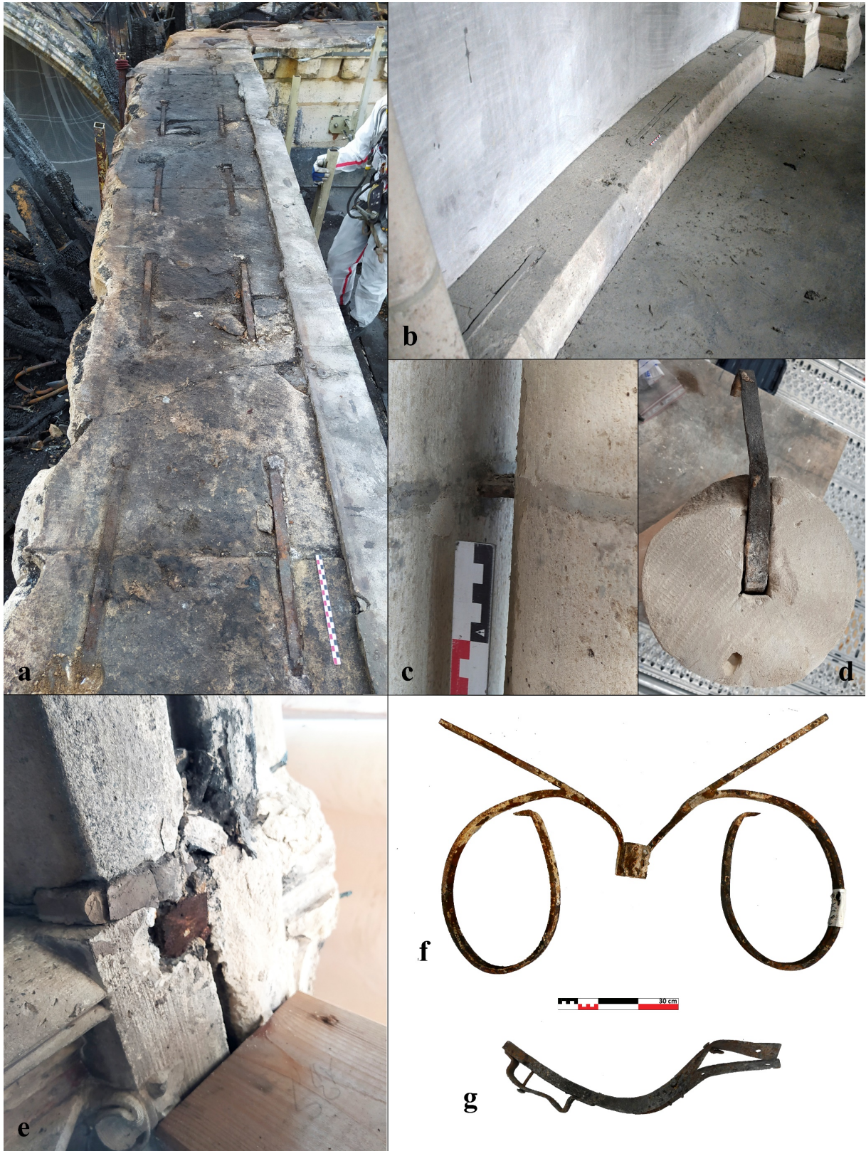
Figure 2 : Iron armatures in Notre-Dame de Paris. (a) Cramps discovered on the top of the upper walls (b) cramps in the tribunes (c) & (d) cramps attaching monolithic column blocs to the piers in the nave (e) ancient iron bars remains in the upper bays (f) iron armature of lead cresting (g) iron armature of spire lead decoration
