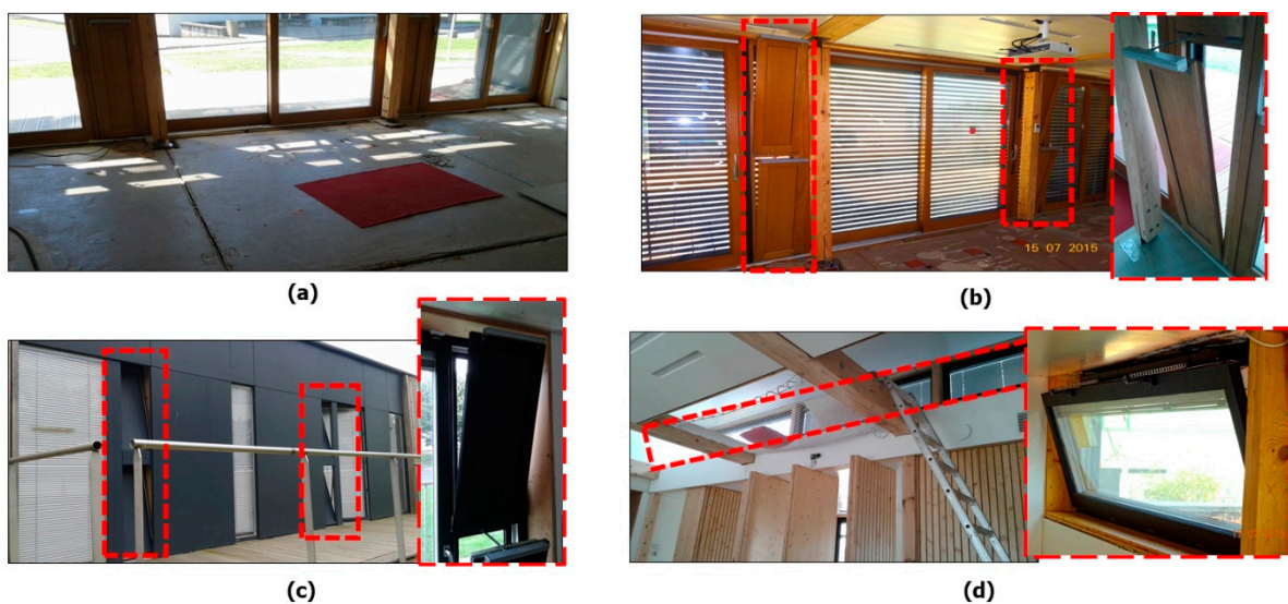
Figure 1. Architectural features: (a) floor concrete slab, (b) programmable solar shades and natural ventilation openings (inside red squares) on the south glazed façade, (c) the north facade, (d) and the shed roof.
