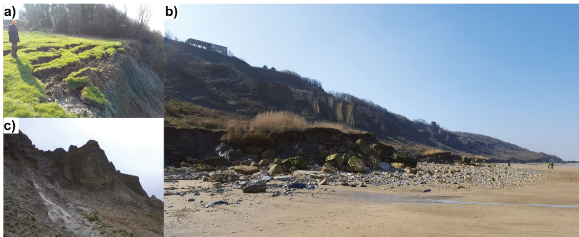
Fig. 2 a Clues of future rotational slidings at the main scarp surface (up to 70 m height), involving limestone rockfalls underneath Coral Rag. b Leakages that take their source at the grey marl Cenovian top layer, triggering mud and rock slidings forming the basal scarp at the VNCs toe. c Housing threatened at the top. Pebbles, fossils and
