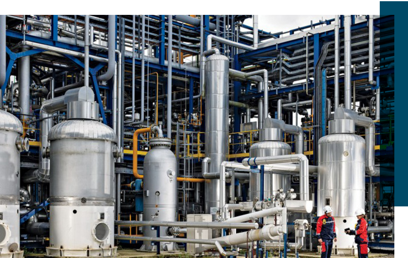
Air Liquide's Cryocap CO 2 -capture technology is in use at its hydrogen plant in France – Credit Air Liquide
