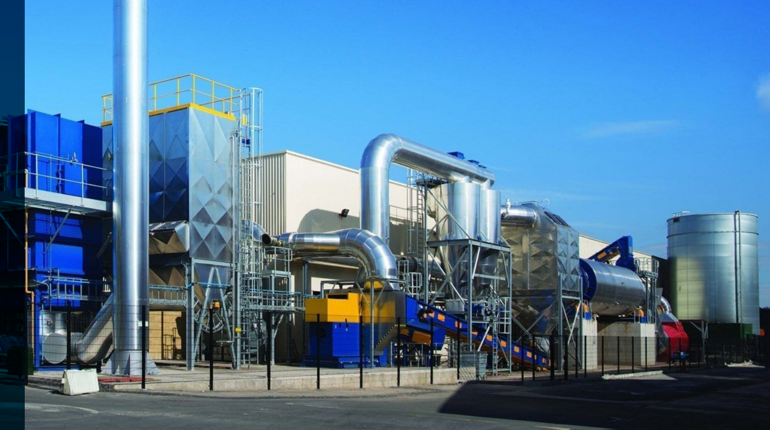
EQTEC Plc 1.1 MWe Market Development Center (MDC) turning biomass waste into hydrogen energy, biofuel and electricity (Italy) – Credit: energynews
