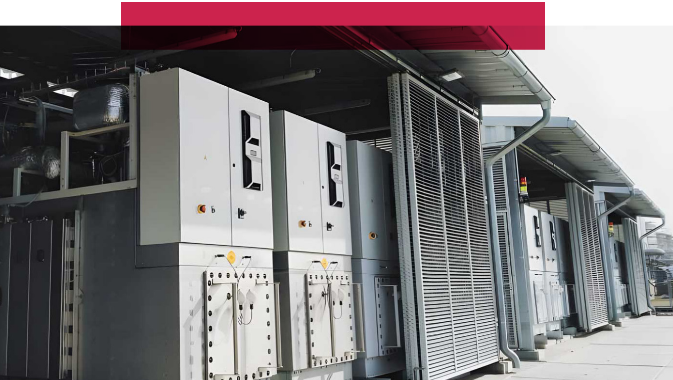
MultiPHLY project in Rotterdam, Netherlands. Multi megawatt SOEC electrolyser for the production of green hydrogen – Courtesy of Sunfire.
