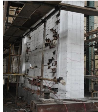
(b) back view of wall collapse
