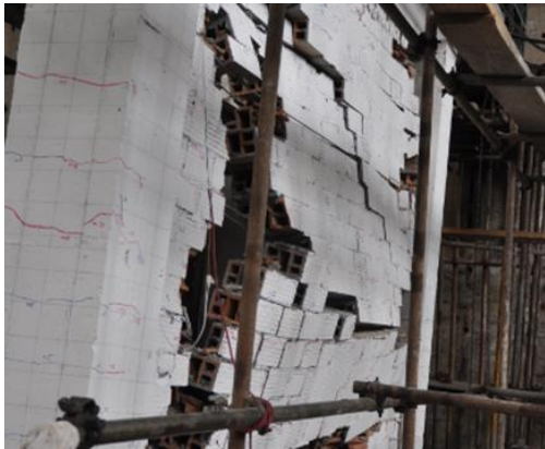
(a) front view of wall collapse
