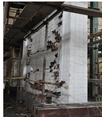
(b) back view of wall collapse
