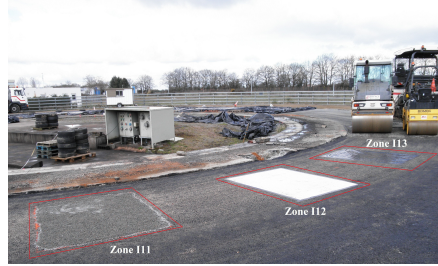
(a) 25 m track with artificial defects before laying the wearing course layer. 'Zone 113' indicates Tack-free based defects (Zones 111 and 112 are respectively Geotextile and Sand-based defects)
