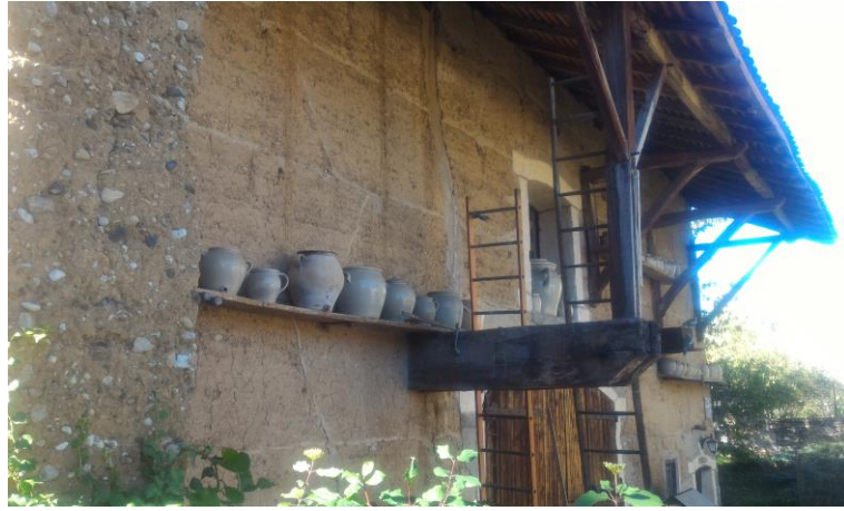
Figure 1: Rammed earth house in the village of St. Chef, Iserre, south of France.
