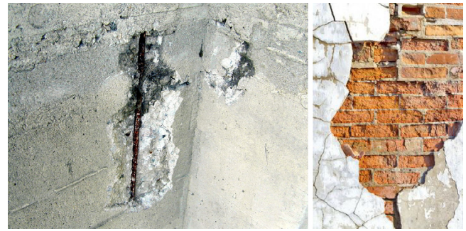
Fig. 4. Two real examples of weathering effects of water and rust on a building facade.
