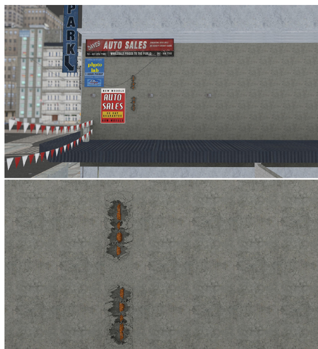
Fig. 13. A building with a visible rusting iron pipe exposing concrete and the pipe itself, top: from a distance view; bottom: closeup view.
