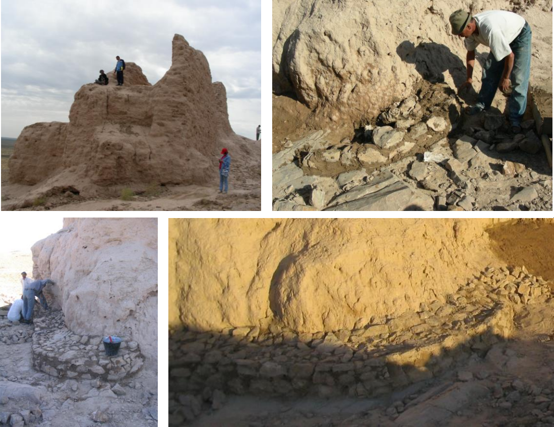
Treatment of the exit zones of the water flows on the eastern side of Ayaz Kala with addition of a embankment made of stone masonry along the most affected wall
