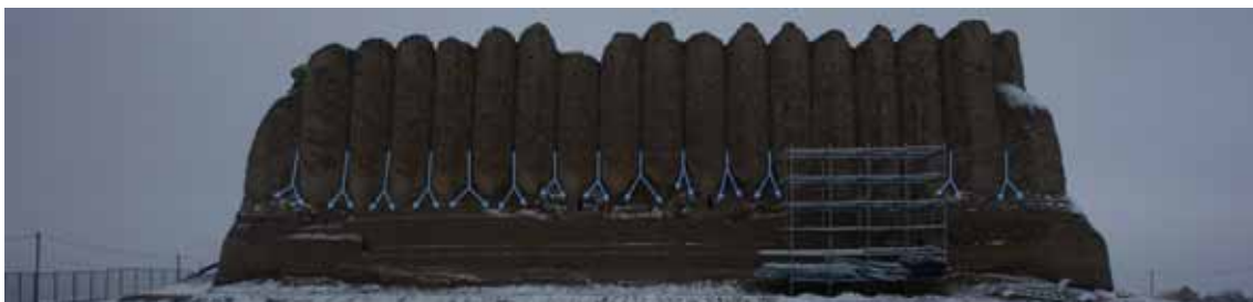
Erosion process at the bases of the corrugatuions
