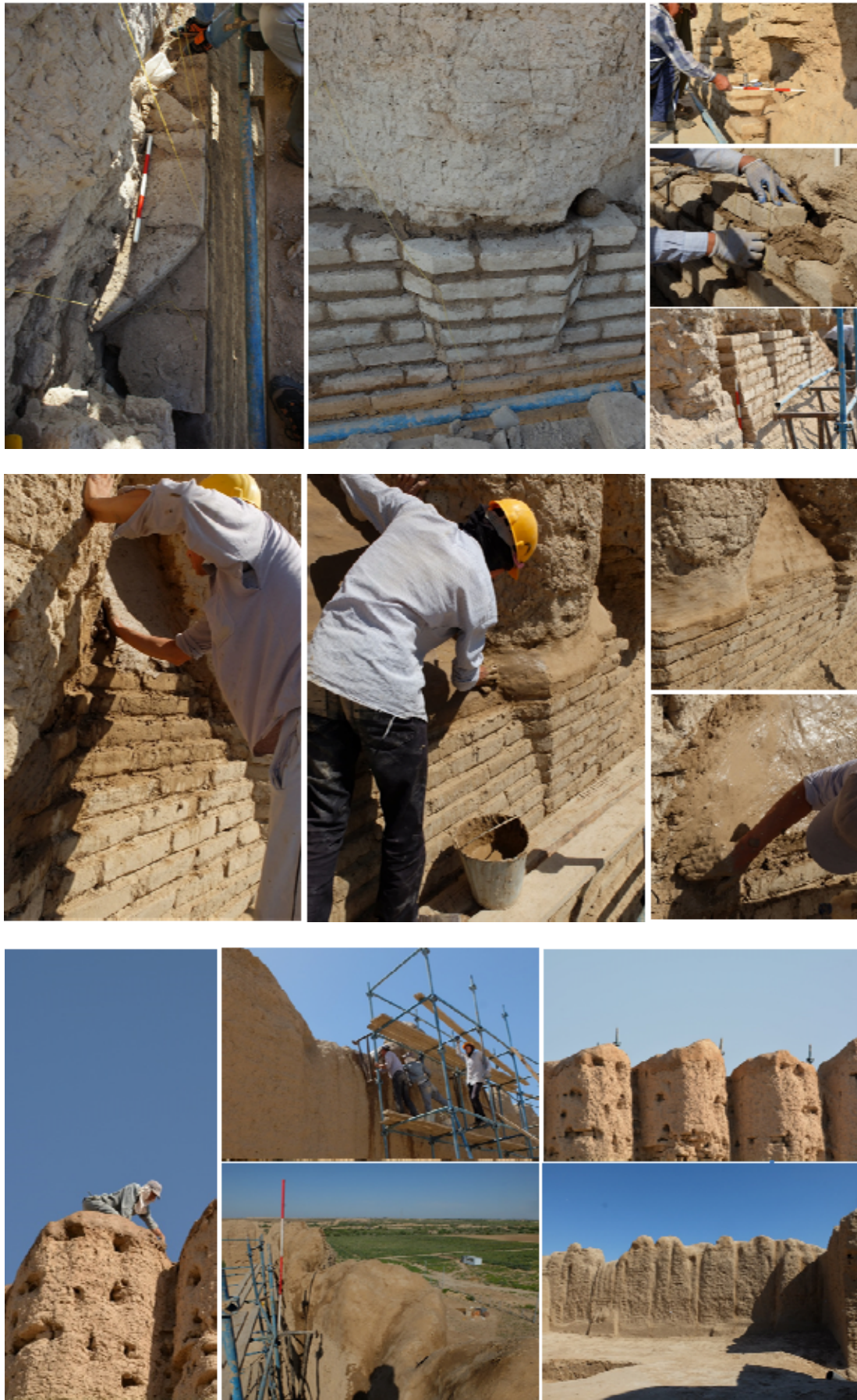
Selection of pictures (1/2). Work in progress on the Greater Kyz Kala in May 2015
