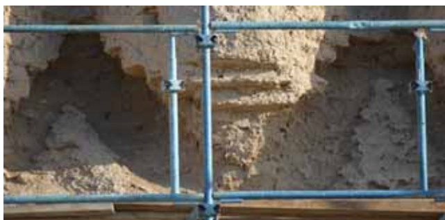
Detail of the erosion (column 10)
