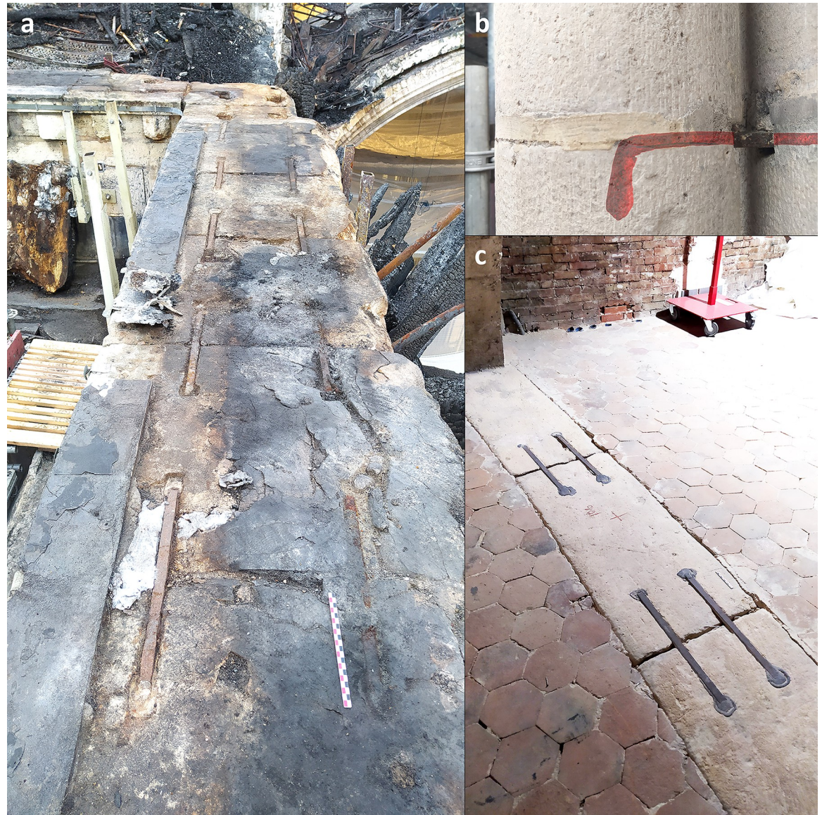
Fig 1. Iron armatures in Notre-Dame. a. Iron staples of the top walls (southern nave looking on the angle of the southern transept). b. Iron staples inside the monolithic columns of the nave (view of the staple in red). c. Iron staples in the tribunes of the choir (staples n° 121 to 124).
