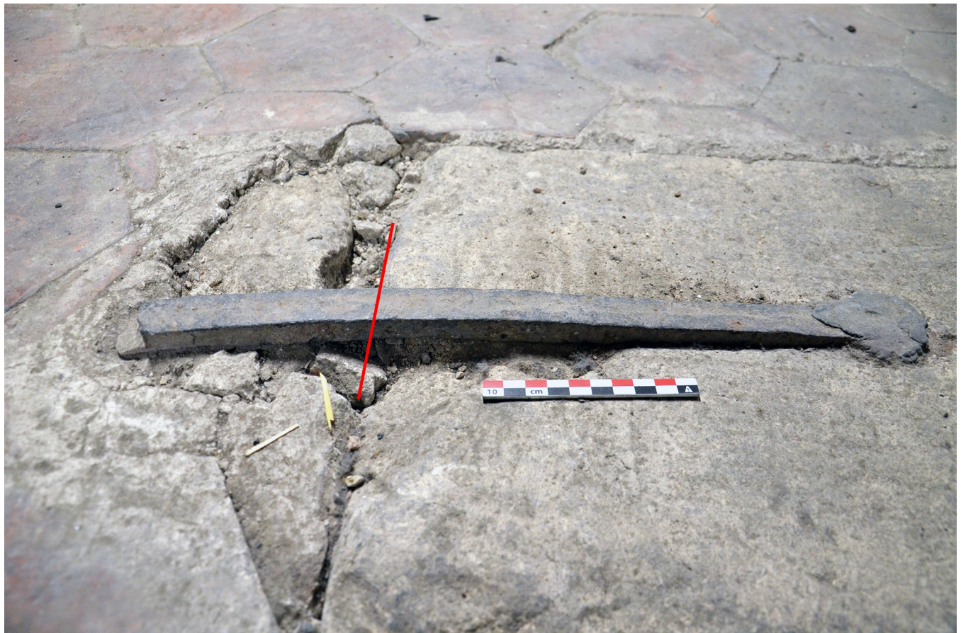
Fig 6. Broken staple in the tribunes (TRIB01S). The red line indicates the sampling. The sample was then cut longitudinally for analysis.
