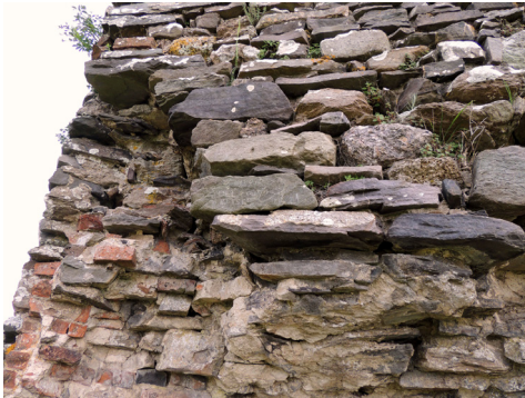
Fig. 6- The small, roughly hewn ashlar of grey to green-purple quartzite constituting most part of the perimeter walls (photo by Fabio Fratini, 2022)
