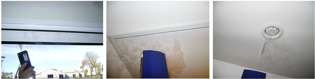
8 Fig. 2. Examples of leakage detection by a smoking device, from left to right: leakage through the 9 frame of a sliding door (leakage C6, strong), leakage through attic trap door (leakage E2, medium) 10 and leakage through ceiling downlight (leakage F5, strong).
