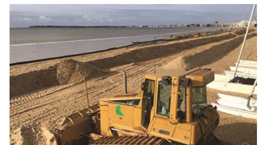
Fig. 4. Work for the creation of the Ecoplage, on the beach of La Baule, January 2019.
