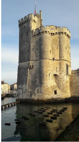
Fig. 10. At high tide of low coefficient, the top of the walls remains in the open air.
