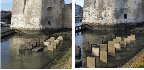
Fig. 9. During the tide's descent, the bottom of the walls remains a longer time immersed.
