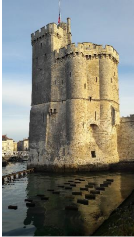
Fig. 10. At high tide of low coefficient, the top of the walls remains in the open air.
