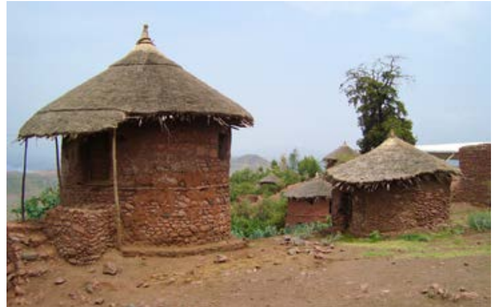
A Tuluk is a round, two-level house, built of stone and earth walls. The example above shows that the earthen plaster covering the wall is almost gone © Ishanlosen Odiaua
