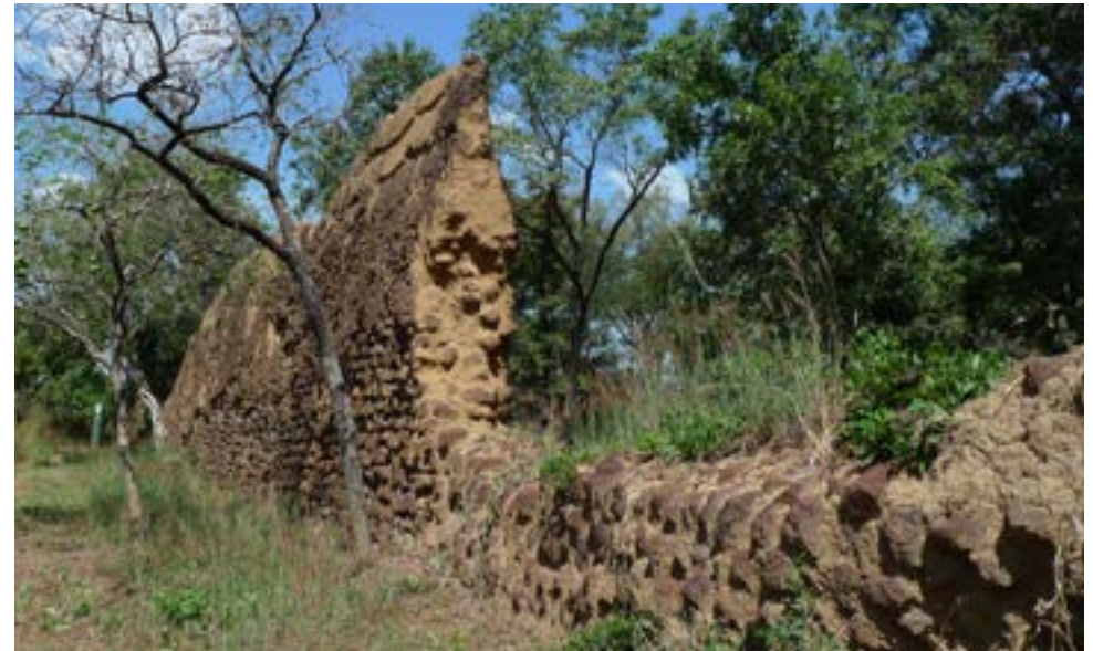
Tear on west wall © David Gandreau, CRAterre
