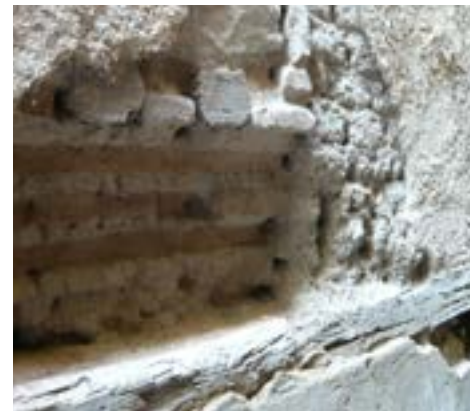
Detail of degraded plaster and of the earth bricks showing underneath © Jean-Marie LeTiec, CRAterre
