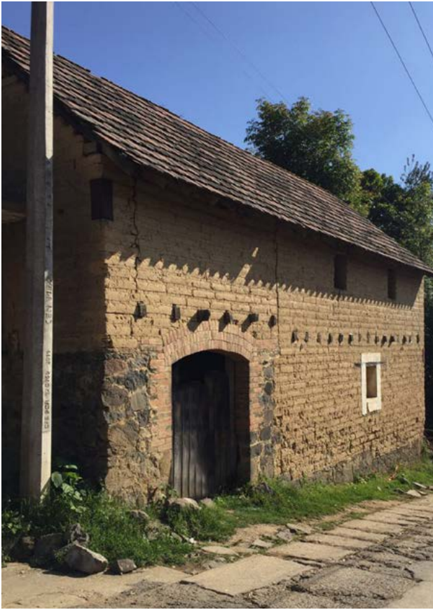
Fig.4: Roofs & attics fulfill several essential functions within the built system. Tetela, Morelos
