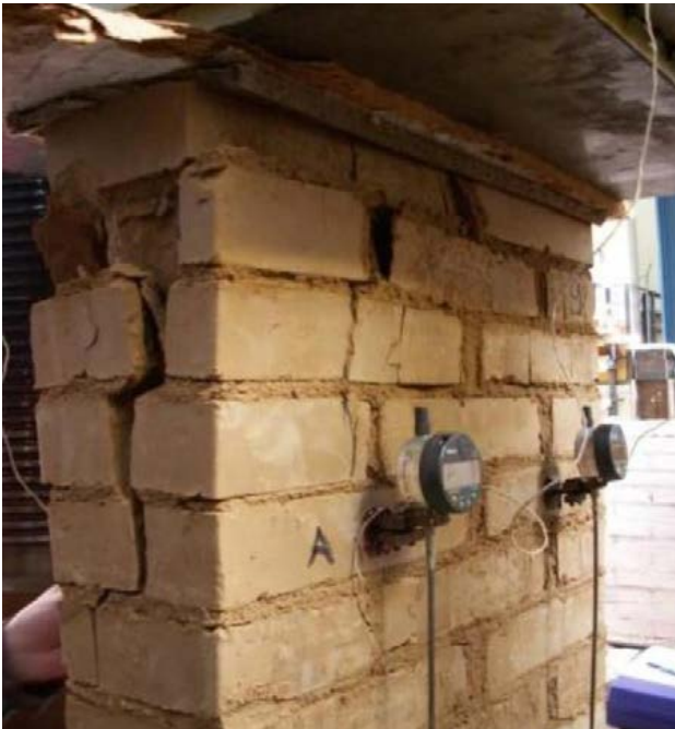
Fig.4: 600/150/900mm pillar failure cracks at mid-width and mid-thickness accompanied by other faults. Various wall sizes, clay materials, walls bonding pattern and the influence of moisture content were tested during the research.
