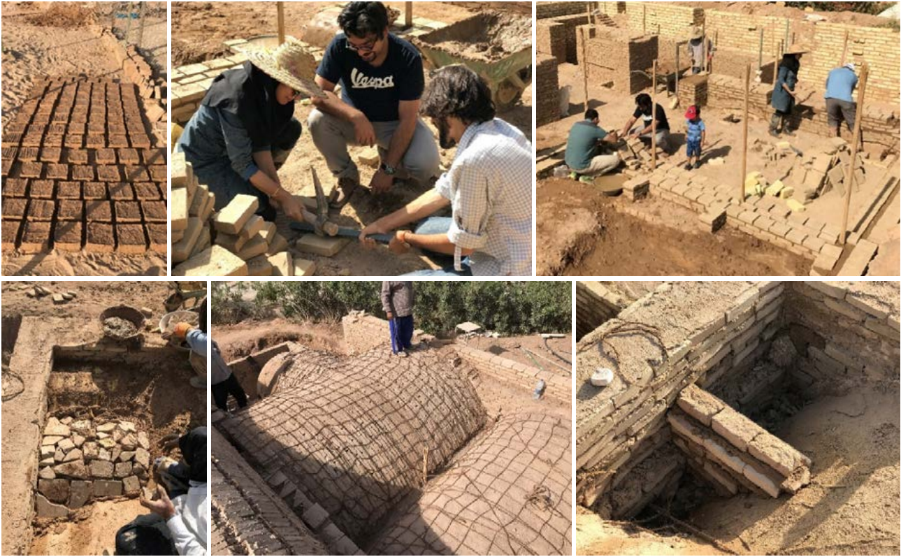
Pictures 4, 5 and 6: Students practical experience with earthen construction Pictures 7, 8 and 9: Structural reinforcement by sazoo mesh and konoo technique for thermal and structural purposes
