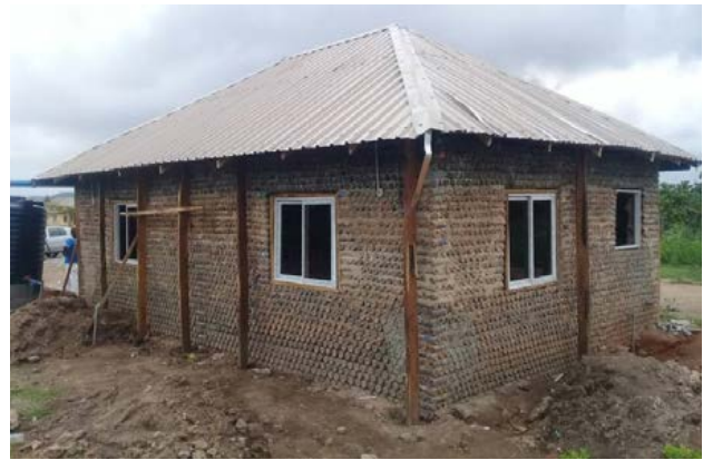
Fig.5: The DMU-IESD's low impact housing using earth and recycled plastic bottles, Mpape (Païpe), Abuja-Nigeria
