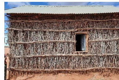
Baraako are left unplastered in hotter regions to allow easy ventilation, better insulation and comfort – Doolow, Jubaland – CC Enrique Sevillano Gutiérrez, CRAterre
