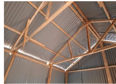
Imported squared timber and CGI sheets are used in recent constructions. Doolow, Jubaland – CC Enrique Sevillano Gutiérrez, CRAterre
