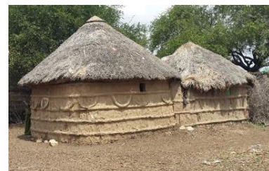
Mundul . The maintenance of these constructions and other vernacular typologies is mastered by their inhabitants – © Shelter Cluster Somalia
