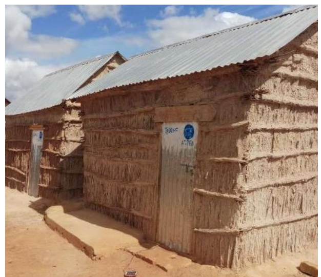
Baraako Transitional shelter – © Shelter Cluster Somalia
