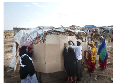
Mutual support for the construction of a buul in an IDP Camp in Garowe, Puntland – © NRC
