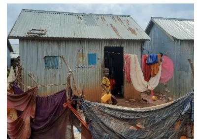
Bioclimatic comfort inside CGI sheet houses is nonexistent. Baidoa, South West State – CC Enrique Sevillano Gutiérrez, CRAterre
