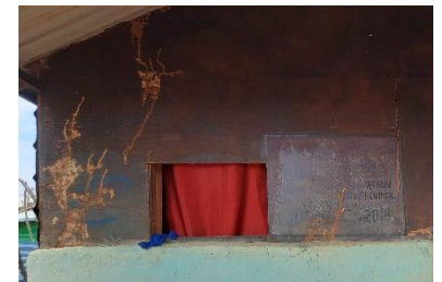
Plywood panels used in some hybrid shelters are very easily attacked by termites. Doolow, Jubaland – CC Enrique Sevillano Gutiérrez, CRAterre
