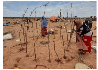
Construction of the structure of a buul in Doolow, Jubaland – CC Enrique Sevillano Gutiérrez, CRAterre
