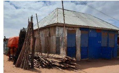
CGI construction with hip roof in Doolow, Jubaland – CC Enrique Sevillano Gutiérrez, CRAterre
