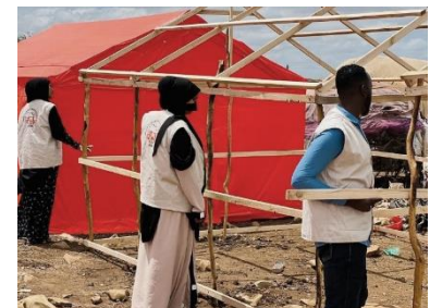
Timber structure of an Emergency Shelter Kit in Baidoa – © UNHCR / African Volunteers for Relief and Development
