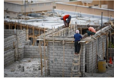
Construction of a reinforced concrete structure with hollow blocks infill in Mogadishu – CC UN Photo / Stuart Price
