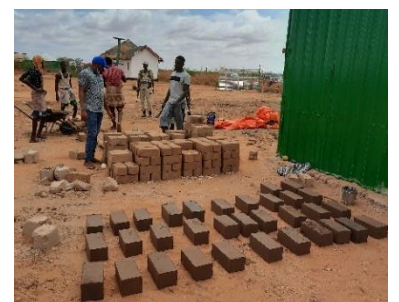
Income generating activities linked to shelter projects can be numerous, from construction to production of materials (Doolow, Jubaland) - CC Enrique Sevillano Gutiérrez, CRAterre
