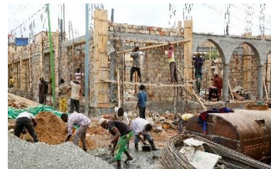
Construction with stone and Reinforced Concrete structure in Baidoa, South West State – CC AMISOM / Abdi Dakane
