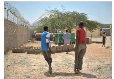
Cement blocks are not a replicable alternative for IDPs. Two persons carrying concrete hollow blocks in Mogadishu - CC UN / Tobin Jones
