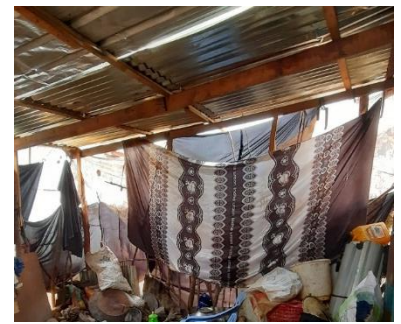
Some families use part of the roof trusses of their main house for constructing extensions. Baidoa, South West State – CC Enrique Sevillano Gutiérrez, CRAterre
