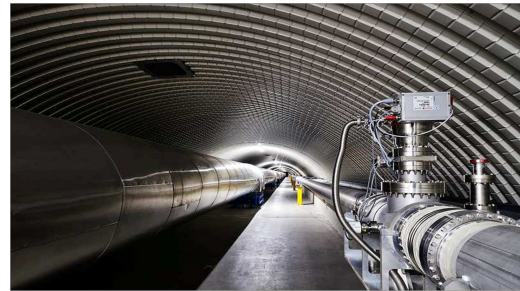
Figure 3. View of the filter cavity for the Frequency Dependent Squeezing.
