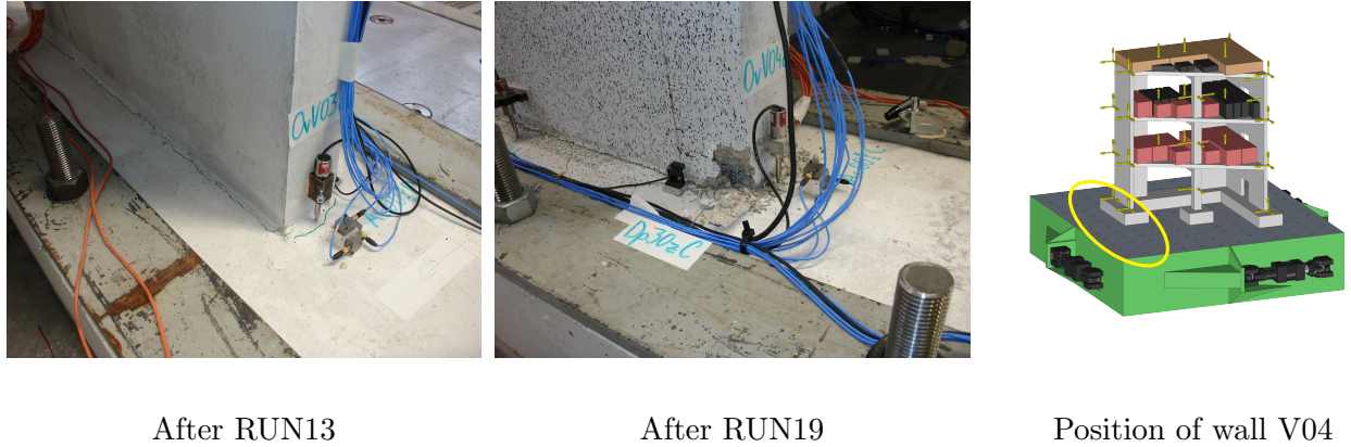
FIGURE 20: Main damage area of the SMART2013 specimen: base of the wall V04. (After RUN13) first crack appearing near the junction between wall and soleplate – sudden rupture of one or more vertical reinforcements. (After RUN19) rupture of the rest of the vertical reinforcements at the base of wall V04 – complete loss of rigidity between wall and soleplate (breathable crack) – high damage level to concrete.
