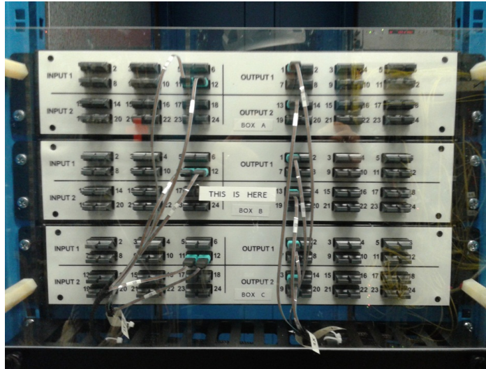
Figure 9.19: Dual 12 \times 12 fibre ribbon remapping modules in a 2U enclosure installed in a standard LHC rack in Point-5. 8 such dual modules will be required on ATLAS.
