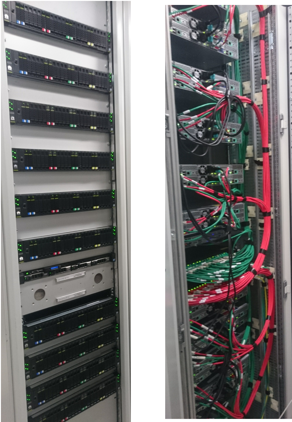
Figure 16.8: Photographs of a typical event processing rack configuration in SDX1 . The left photograph shows the front side of the servers, while right one the rear network interconnections to the rack-level switches.
