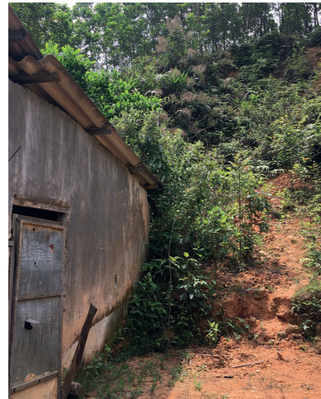
[Figure 11.5] Landslide threaten house
