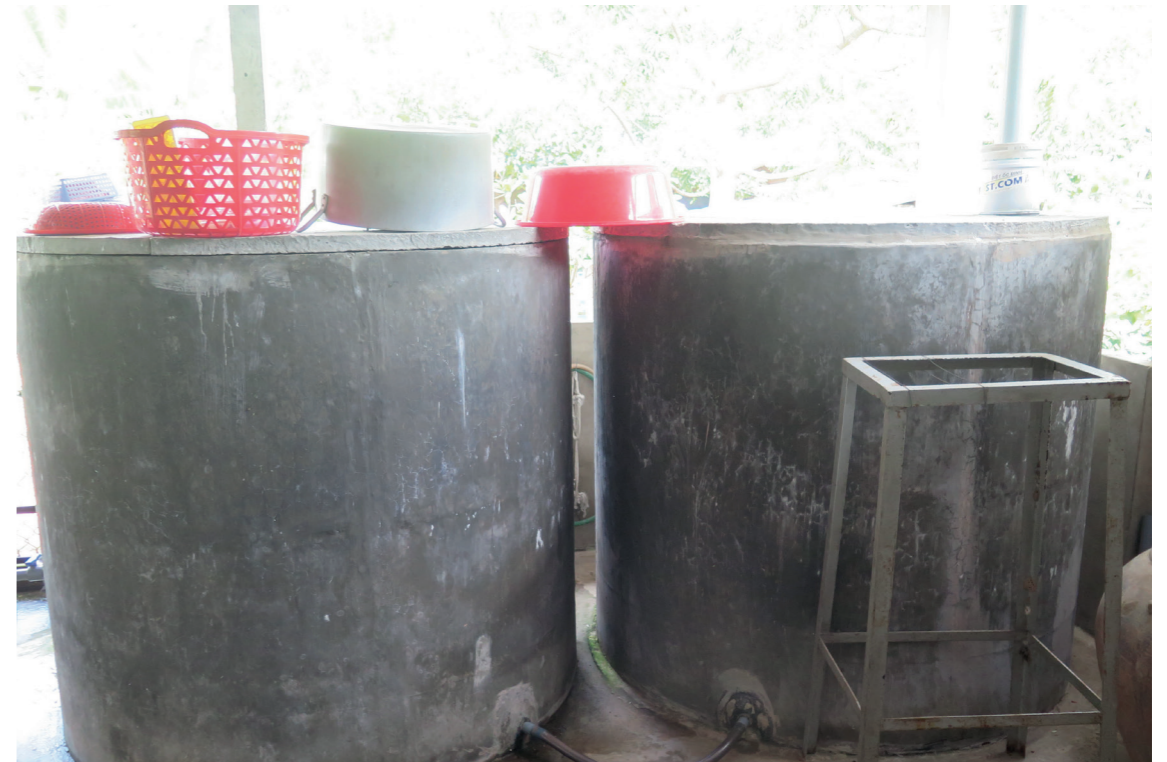
[Figure 11.11] Individual reservoir to stock rainwater Binh Dai district, Ben Tre Photo credit: ©Olivier Tessier
