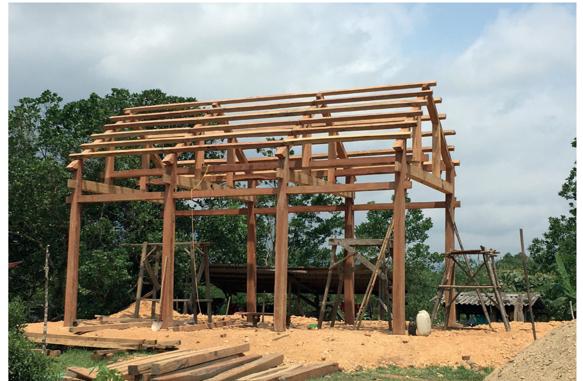
[ Figure 11.9 ] New wooden house building in upper location after flood A Luoi district, Thua Thien-Hue Photo credit: ©Nguyen Cong Thao
