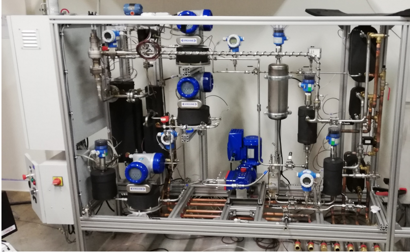
Figure 1. Picture of the pilot plant.
