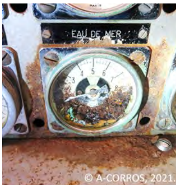
Figure 7. Cadran composite altéré, © A-CORROS 2021.
