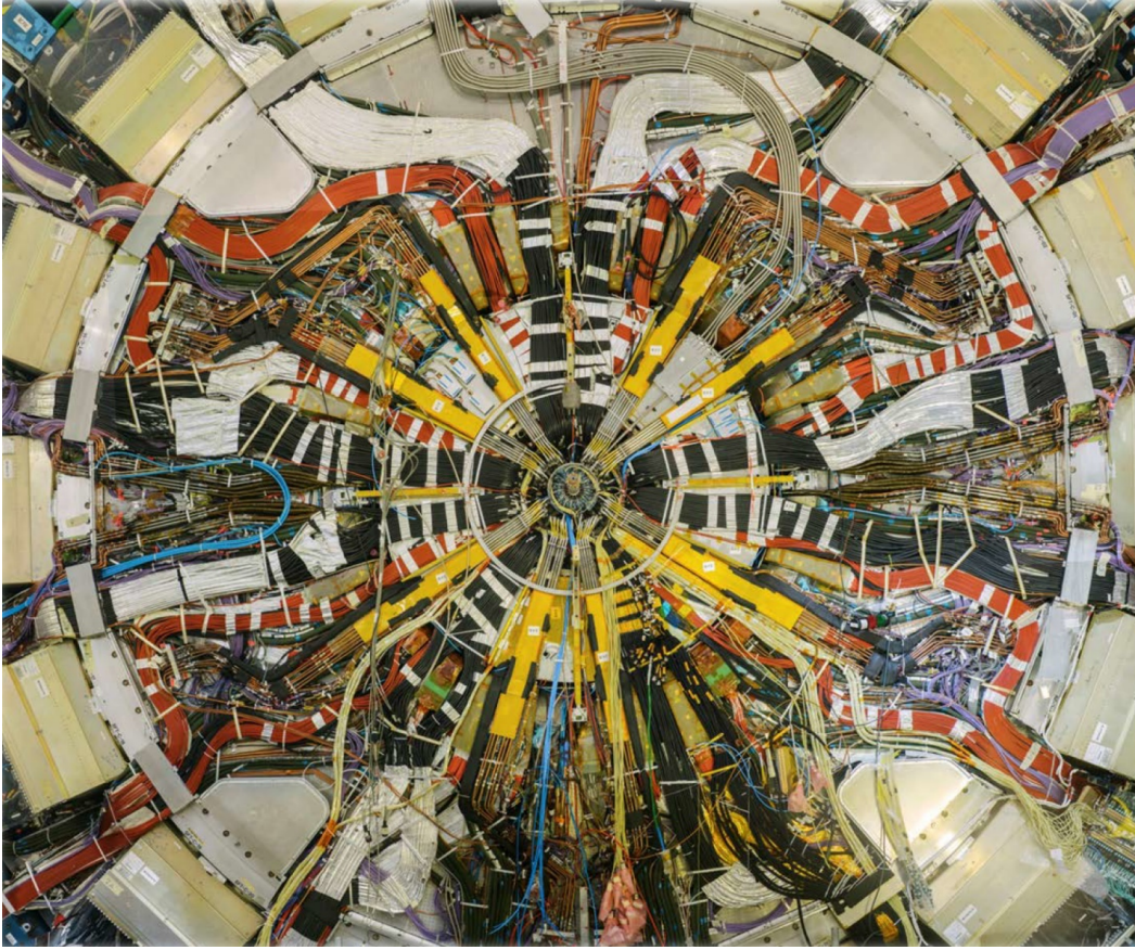
Figure 17.16: Inner Detector services on the Argon Barrel Cryostat wall after installation of the Insertable B-Layer (IBL).
