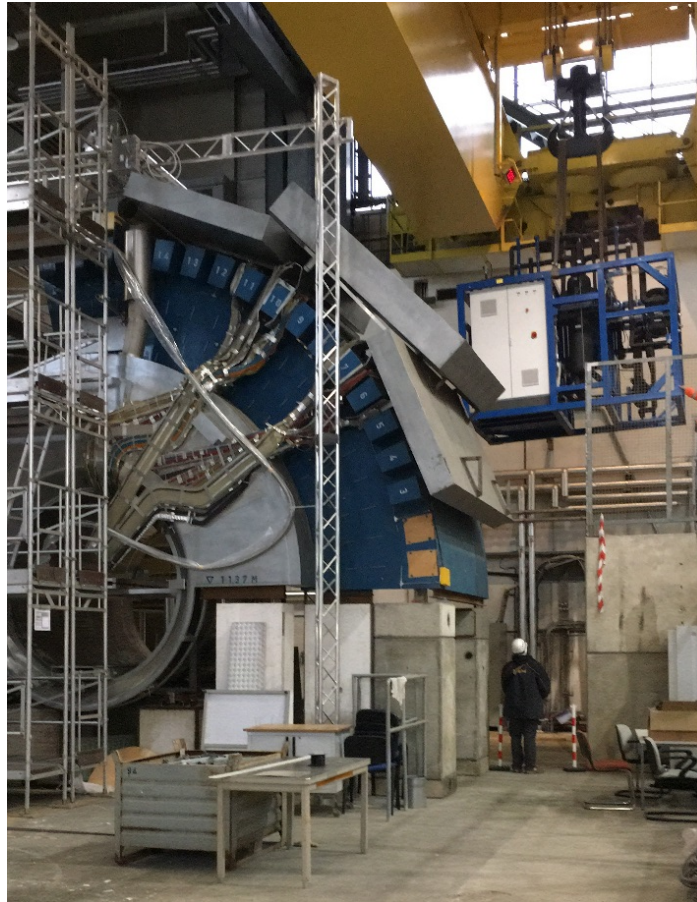
Figure 15.6: Baby-DEMO cooling plant during installation in B180 behind the ATLAS 1:1 mock-up with flex line installed.
