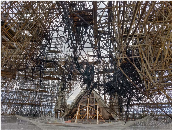
Figure 11. Steel scaffolding (surrounding the spire before the fire) deformed by the high temperatures (photo by Damien Deldicque and Jean-Noël Rouzaud).
