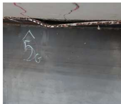
(a). Plastic buckling.
