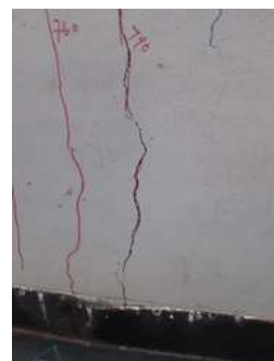
(b). Concrete cracks.
