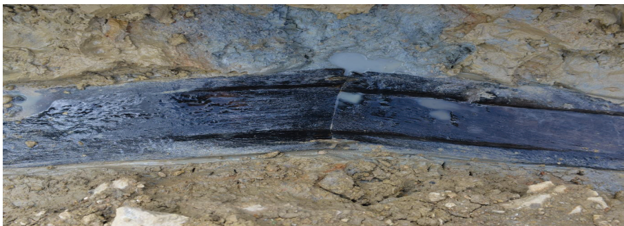
Figure 3. A JUNCTION OF THE WOODEN CHANNEL, WITH AN IRON SOCKET IN THE MIDDLE (A. GOUVERNEUR)
