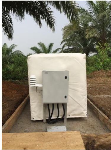
Figure 6: Electrical box which provide energy for the magnetometers.
