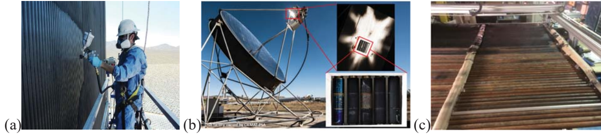
FIGURE 6. (a) Recoating of receiver panel in Ivanpah power plant by BSII, USA, (b) Testing of solar cured absorber samples at CIEMAT’s PSA, (c) Mid-sized automatic coating machine while coating a test panel.
