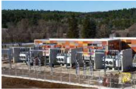
63kV / 15kV substation
