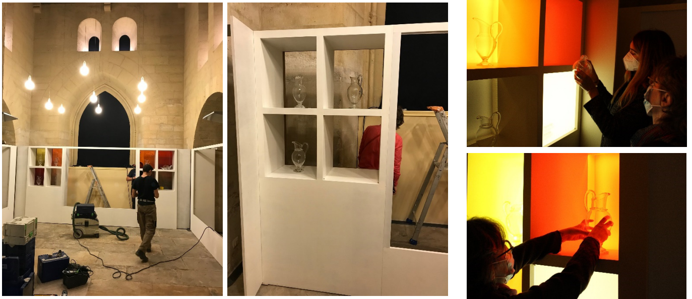
Figure 17. Building up the installation at CNAM.
