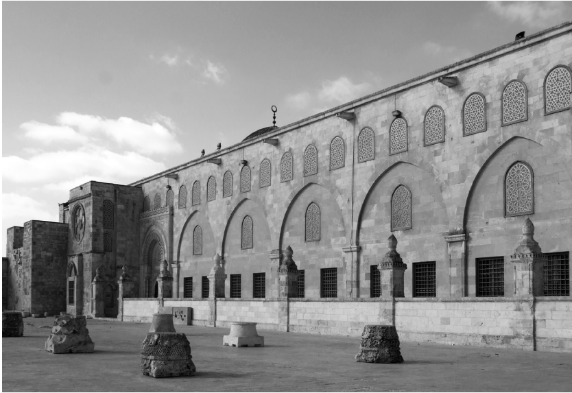
Figure 3.2: The eastern wall of al-Aqsa Mosque, showing the Templar Apse (facing towards the southwest). Photo: Author, September 2013.
