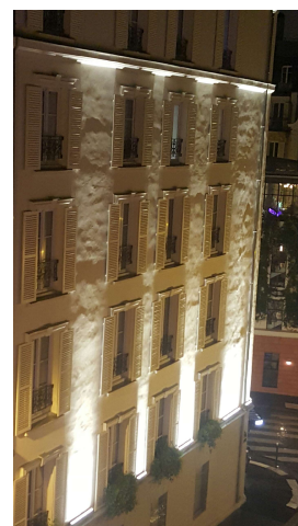
Figure 1. The planarity defects of the facade are highlighted by a grazing lighting, which is the basic principle of RTI.
