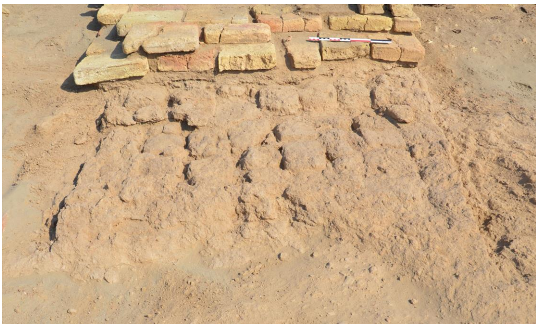
Fig. 10 – Mudbrick Wall 1615 of level II under the north façade of B49 (wall 1575), from the west.
