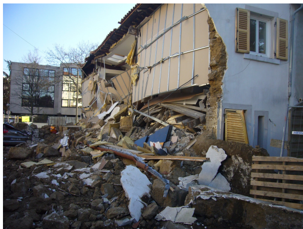
Figure 3. Structural collapse due to inappropriate refurbishment (cement bases, plaster, Rockwool insulation and gypsum board, among others) of a vernacular rammed earth house subjected to water accumulation at the wall base, Lyon, France.
