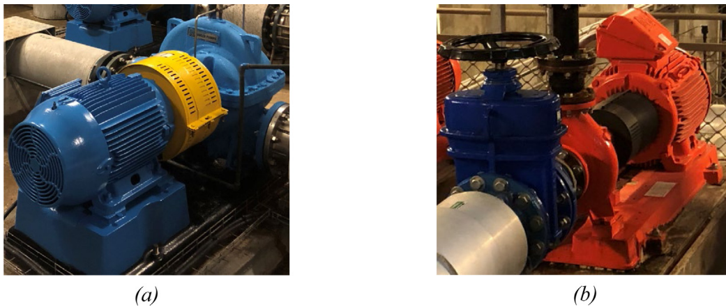
Fig. 5. Primary pump (a) and secondary pump (b).
