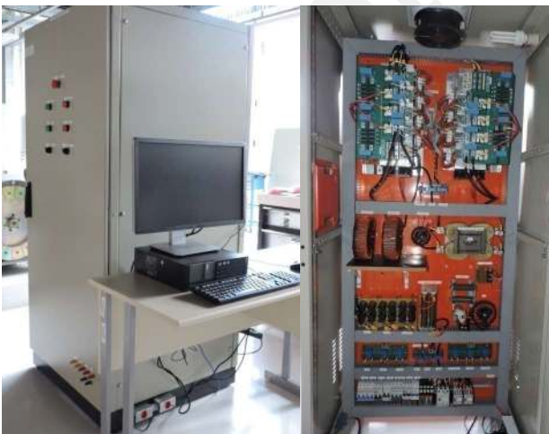
Fig. 7: Converter cabinet of the HRGS.
