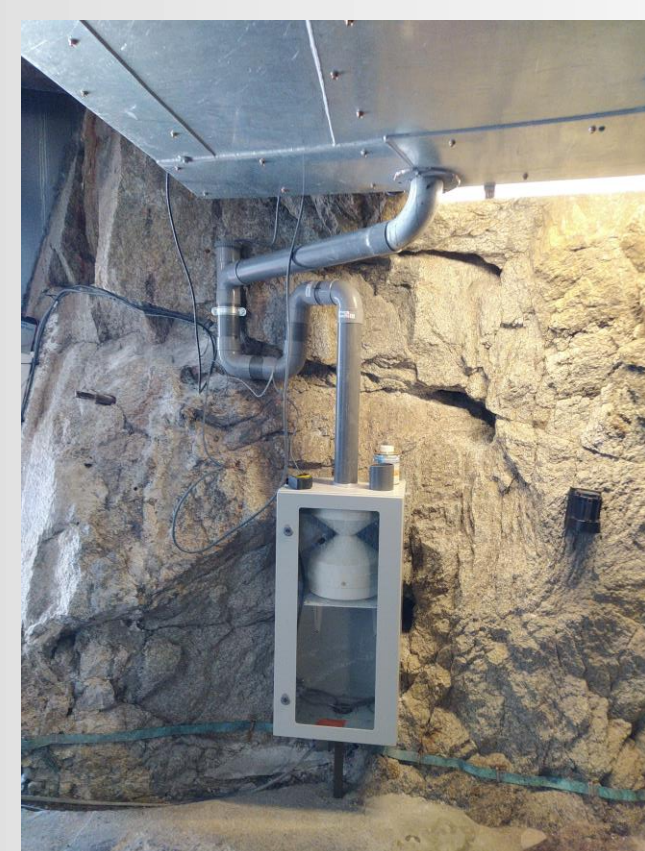
Figure 2A: Snowmelt water monitoring system
