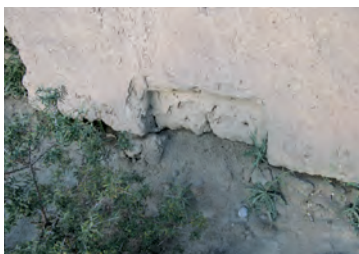
28. Enclosure: recess at the base of the wall in b , 0.6 m wide and 0.3 m high (Q. Devers, 2009).
