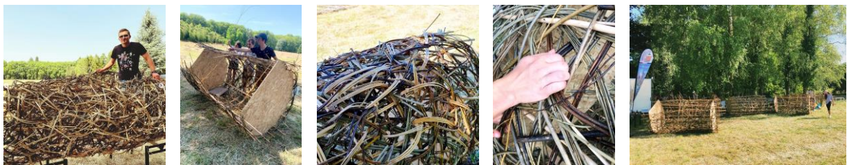
Figure 19: Construction of the footbridge during workcamp I (june-22). The bridge will be finished in august-22.
