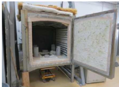
Figure 1 Exterior of electric furnace
